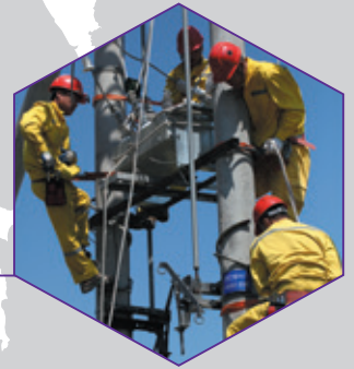
CHINA Oil fields power distribution network automation.
