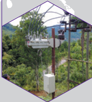
INDIA Power supply quality improvement projects.
