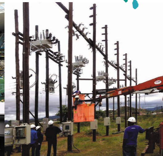
▲ 27 kV outdoor substation with automatic circuit reclosers
