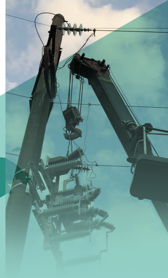
▲ The first installation of Rec35_Smart automatic circuit recloser in Russia
