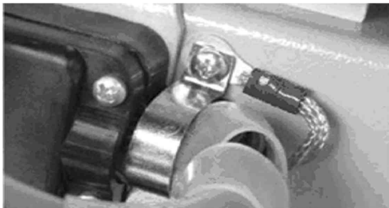
Figure 84 Sample of earthed cable shielding on ISM side
