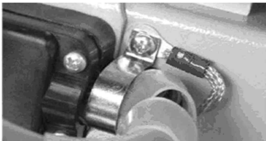
Figure 76 Sample of earthed cable shielding on ISM side
