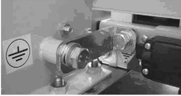
Figure 69 Example of grounding the ISM by copper busbar
